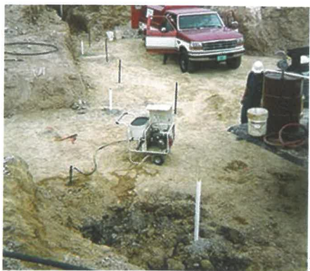
To treat the groundwater contamination at Washington Square Mall, an environmental consulting firm installed temporary wells into which a solution of molasses and water was injected underground.
